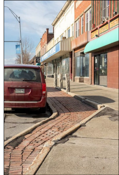
Crumbling infrastructure along Main Street is evident in this photo. Courtesy MaineDOT.
